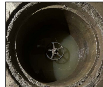
Ground water fills up in the Sump pits due to rain.
